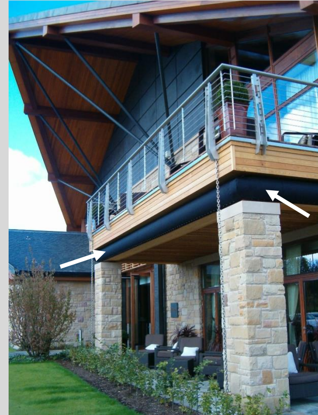
Barrfly™ (arrowed) protecting an outdoor terrace of The Carrick golf club house
